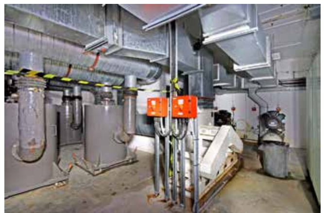
Filter units in the upper level plant room
